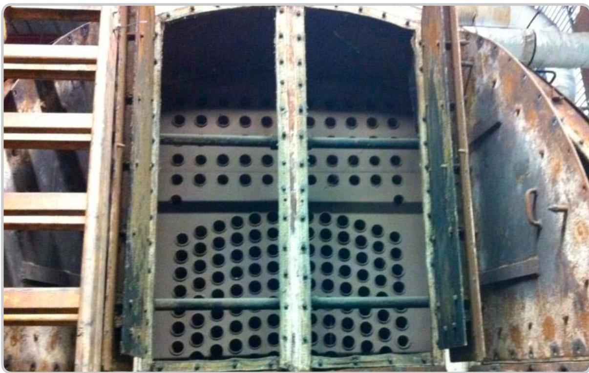
Figure 1: Fire-tube boiler heat exchanger at University College Dublin
